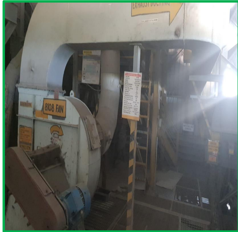
Exhaust fan at Bag house
