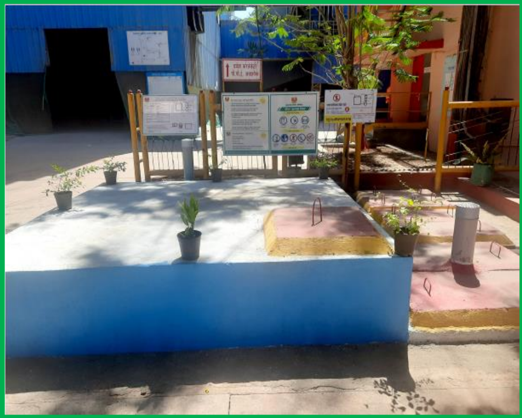
Rain Water harvesting installed in Plant & Jetty to save power for water Re generation
