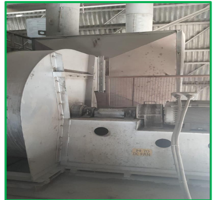
After commissioning. Power Saving 2.7 KWH
